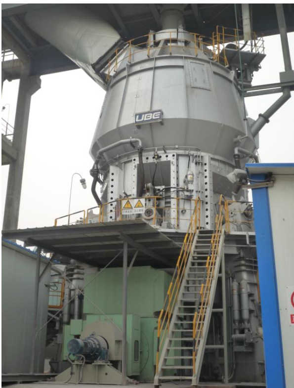
Fig. 4 Slag Grinding Plant and 6 Roller Mill
